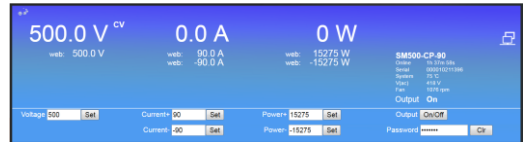
fig 8 - 1 Front console for setting of the output and monitoring various parameters.
